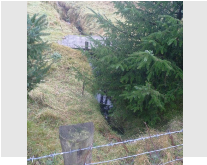
Figure 3-23 View downstream of existing culvert in local road along connection cable route for connection Option to permitted 110kv Lenalea Substation
