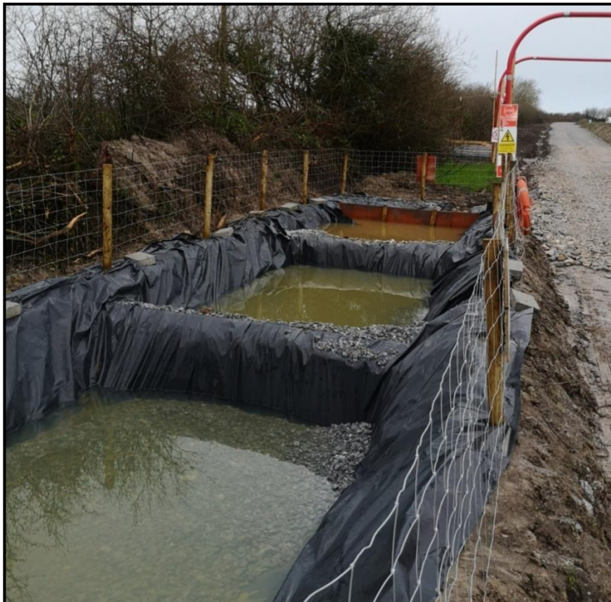
Figure 3-29 Multi-tiered settlement pond with stone filter
