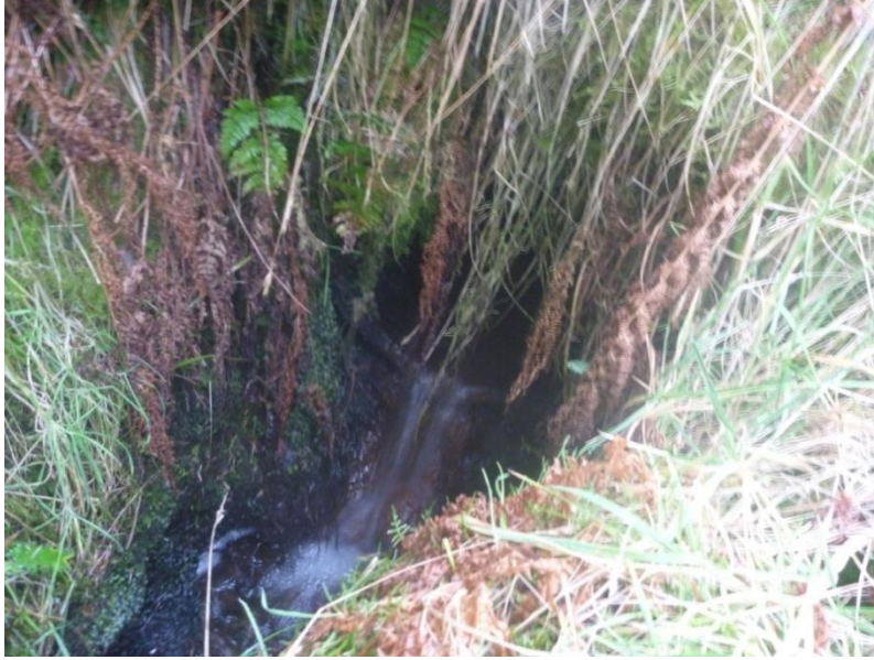
Figure 3-22 Existing culvert under local road along connection cable route for connection Option to permitted 110kv Lenalea Substation
