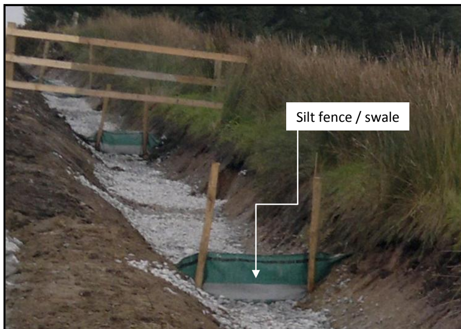
Figure 3-31 Example of a silt fence used in conjunction with check dams along roadside drainage channels
