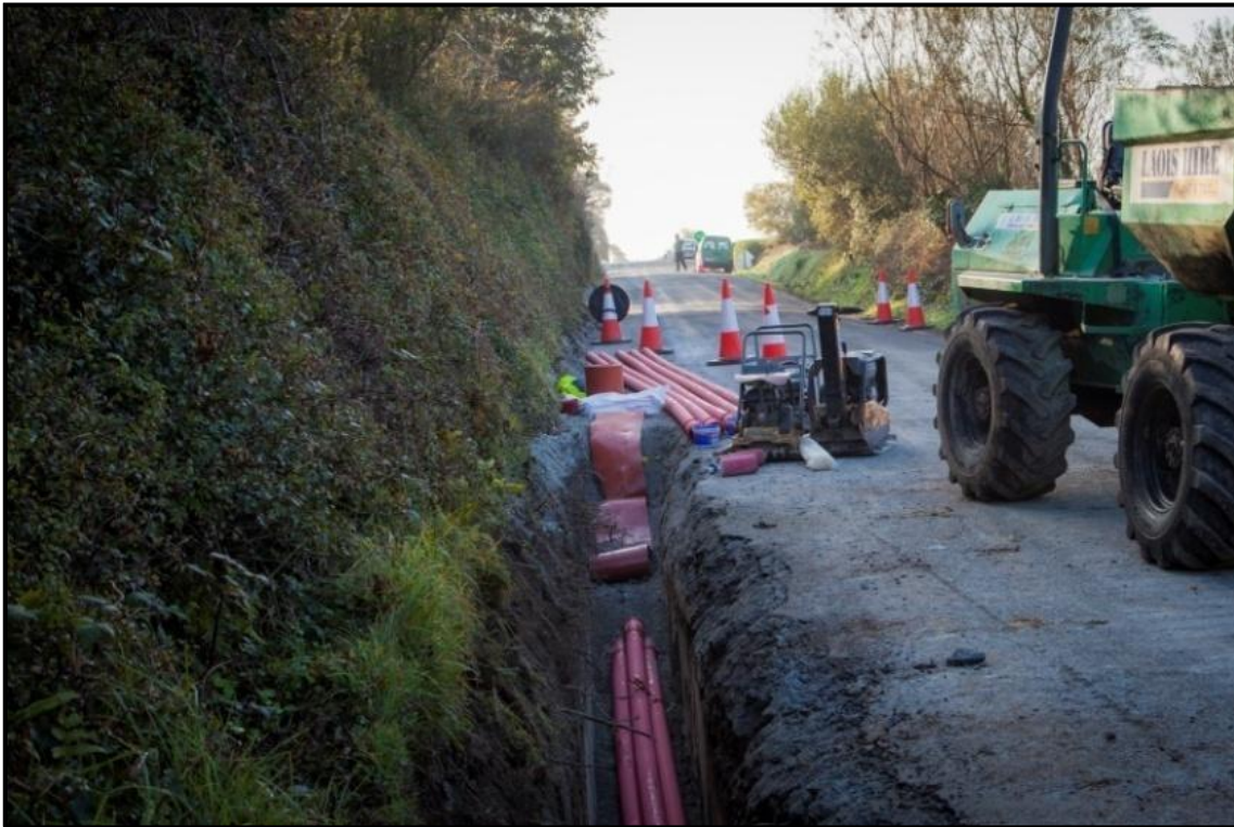
Figure 3-11 Typical ducting installation works for a grid connection cable trench on public road
