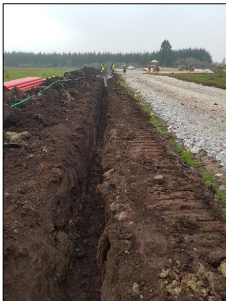
Figure 3-13 Typical excavation works for a grid connection cable trench within wind farm
