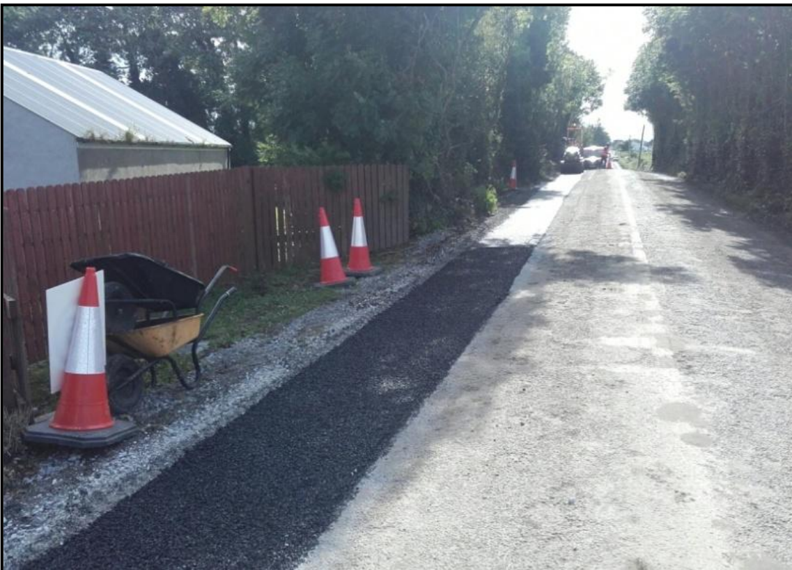
Figure 3-12 Typical permanent reinstatement works for a grid connection cable trench on public road
